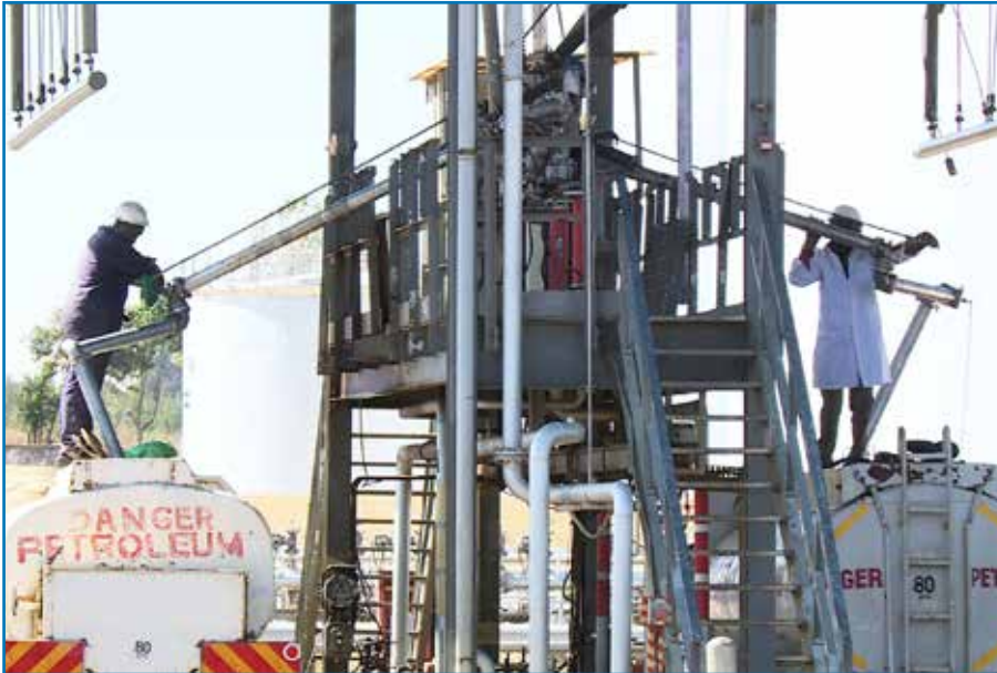
Top loading facility at PS 27 - Eldoret.
