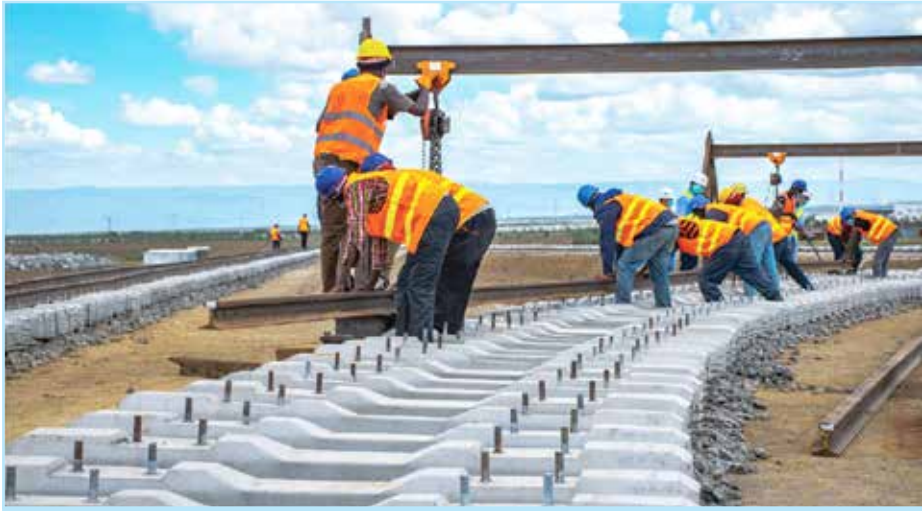
Construction of the railway line linking Naivasha ICD and Longonot railway station.
